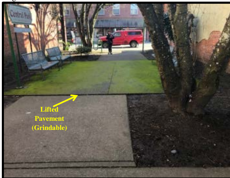
Photo 1. Lifted concrete slabs in the Central Park area of downtown Centralia. View looking east.
