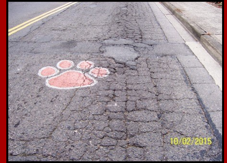
Deteriorating asphalt—Johnson Rd.
