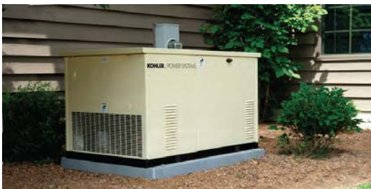
Permanently Installed Generator
