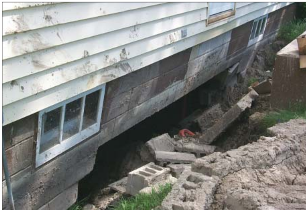
This collapsed foundation wall, caused by heavy floodwaters, constitutes "substantial damage."
