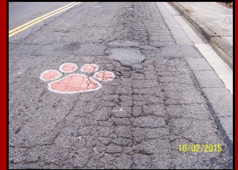
Deteriorating asphalt—Johnson Rd.
